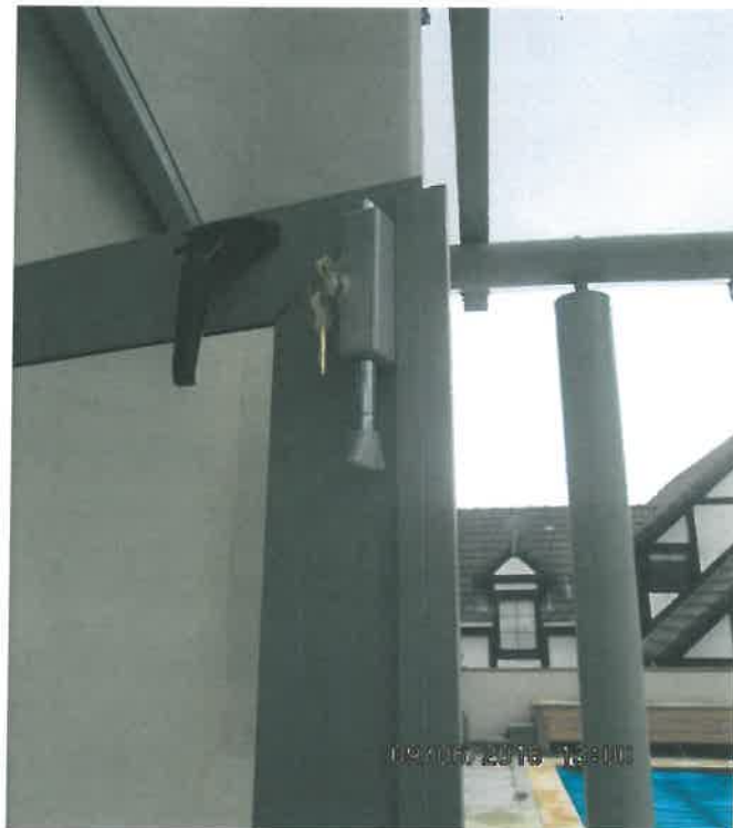
Lockable top bolt fitted to other door
