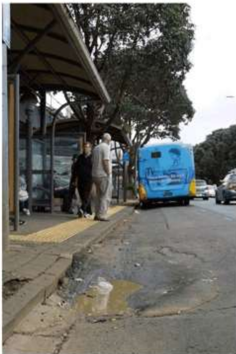
Figure 3 Large pot holes that have been filled with hot mix to no avail.
