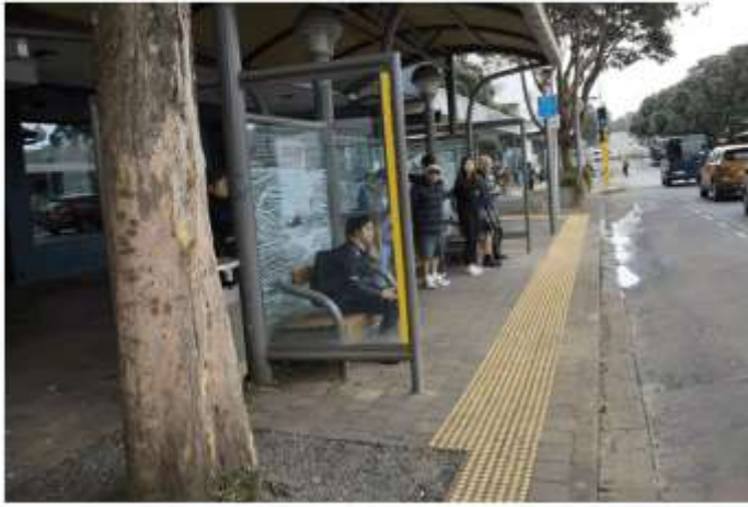
Figure 2 Damaged kerb and channel and roadway sinking outside the main East Coast Bay's loading zone
