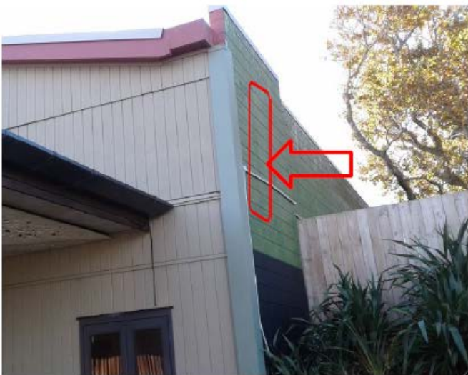
New fire exit through external wall on the south east side of building
