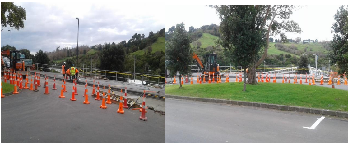
Works near completion at the Meadowbank Train Station. Installation of bus stop and shelter and reconfiguration of on road parking.
