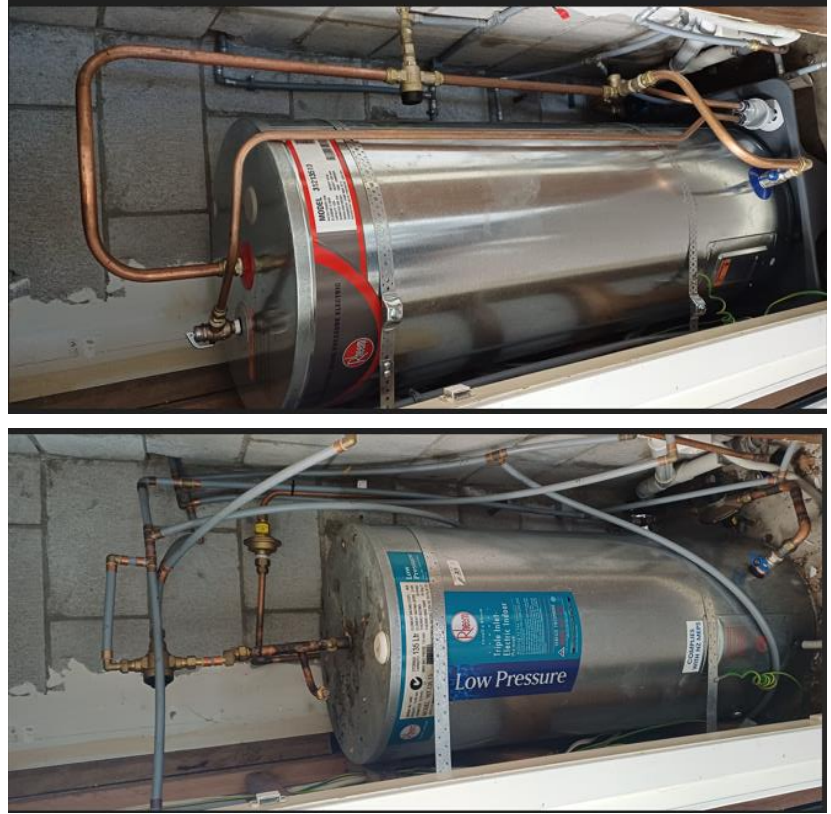
Smiths Ave Community Hall – the water cylinder has been upgraded to code.
